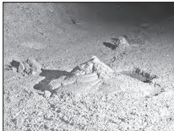
Figure 6: One of many low, dome-and-cone-shaped mounds on the floor that seem to be squeeze-ups from below.
