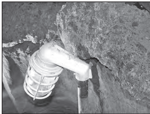
Figure 2: "Jelly Jar" style fixture used in the 1987 re-lighting of the New Entrance and replaced in the current project. Equipped with a 90-watt clear incandescent bulb, these lights grew algae, moss, and even ferns. They also subjected visitors to glare.
